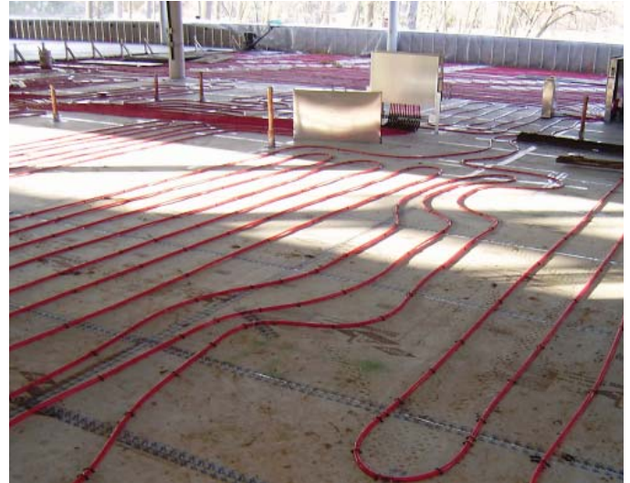
Radiant floor tubing
