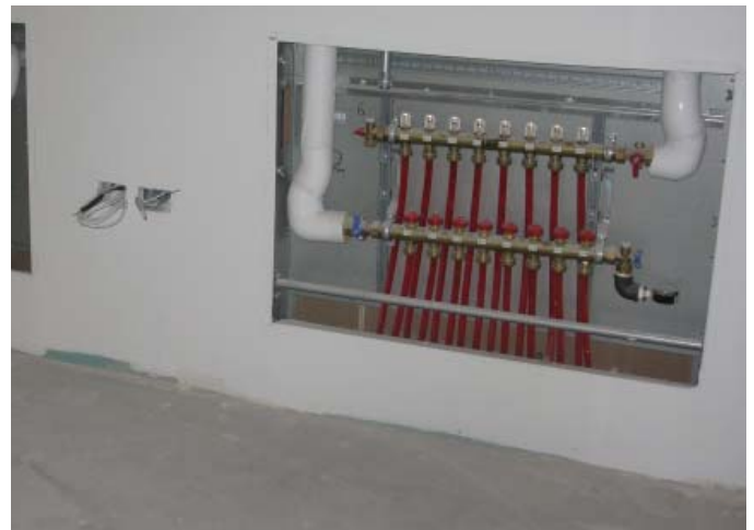
Radiant floor valves
