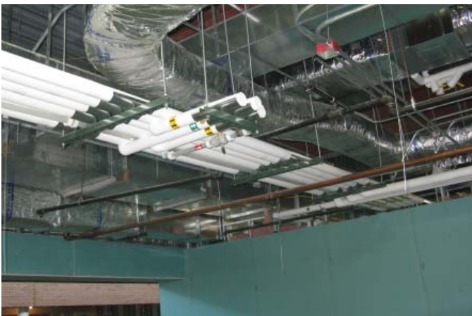
Equipment above ceiling
